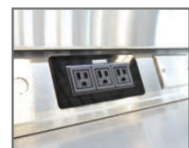
Power feed panels
